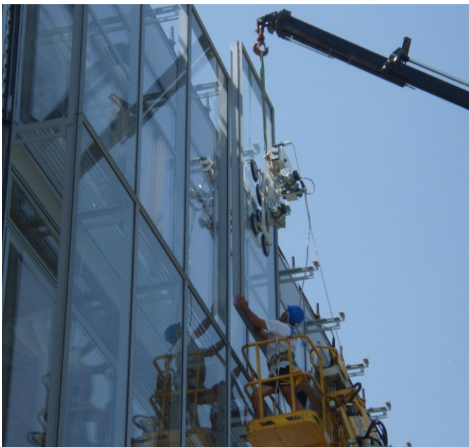
Fig. 9 Maurizio Varratta, iGuzzini Lab , Recanati. Application of the external skin to the main curtain wall, reducing wind pressure and allowing the opening of windows relative to the internal section (even at high levels of the building) © Courtesy of Pichler Projects
