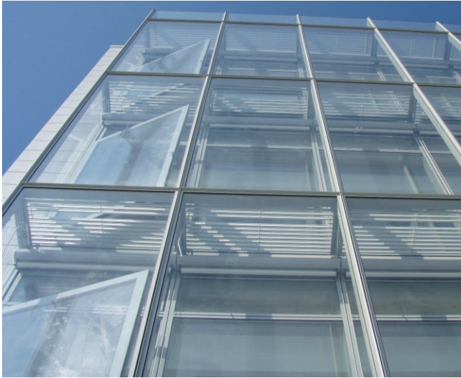
Fig. 5 Maurizio Varratta, iGuzzini Lab , Recanati. Assembly of air flow regulation devices and ventilation louvers, located near the deck sections that are connected to both the external screen and to the internal curtain © Courtesy of Pichler Projects
