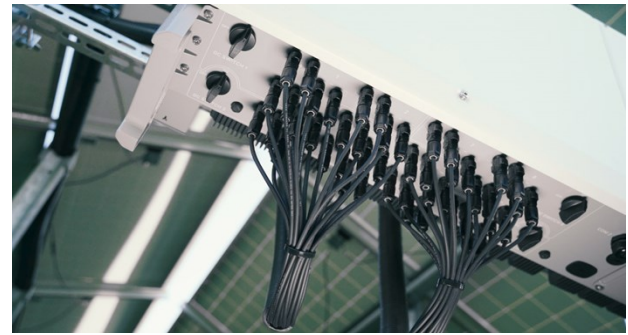
Fig 2. MPPT string cables of string inverter
